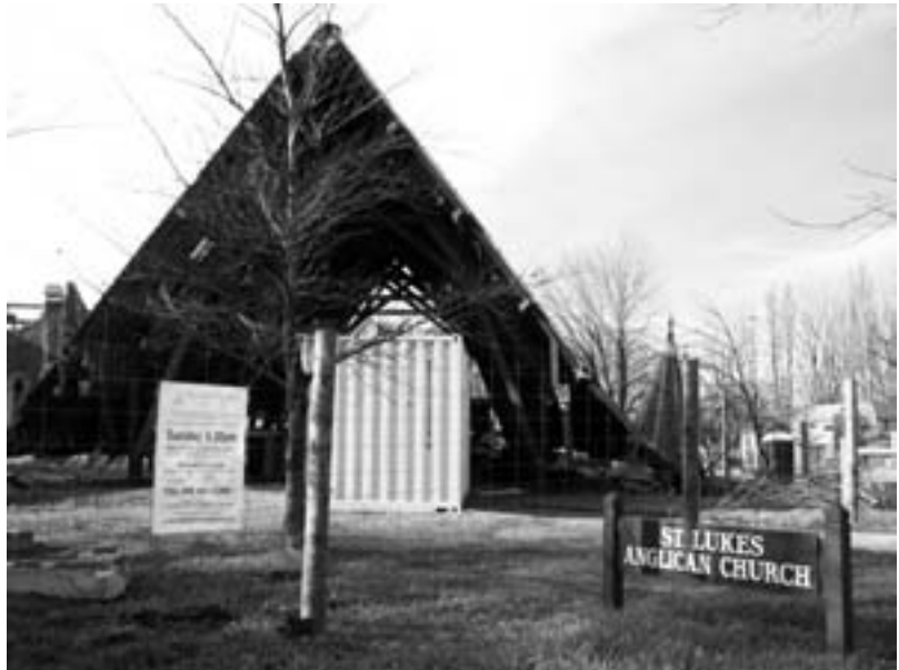
St. Luke's Anglican Church in Christchurch, which was badly hit by the earthquake.
